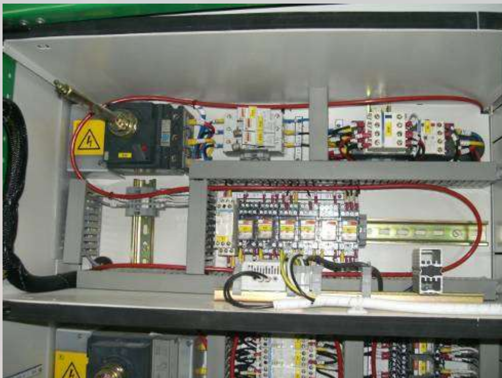
Firetrace system routed throughout the cabinet
