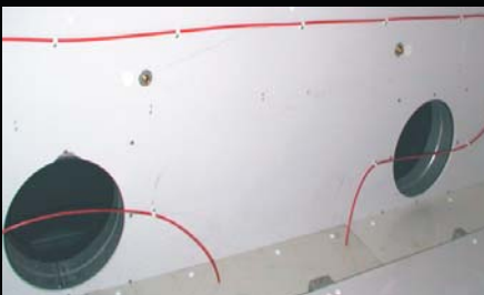
Firetrace detection tubing installed in front of the fume cabinet's exhaust
